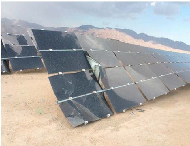
Fig. 4. First Solar's Desert Sunlight section damaged by tornado on July 28, 2015 (source: https://www.ksqj.com/news/solar-farm-damaged-by-desert-center-tornado/62923230 ).
