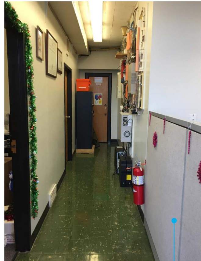
POWER SOURCE WITH NO REDUNDANCIES WITHIN BUILDING ; ADMINISTRATION WORK AREA IS VERY CRAMPED WITH NOT ENOUGH STORAGE.
