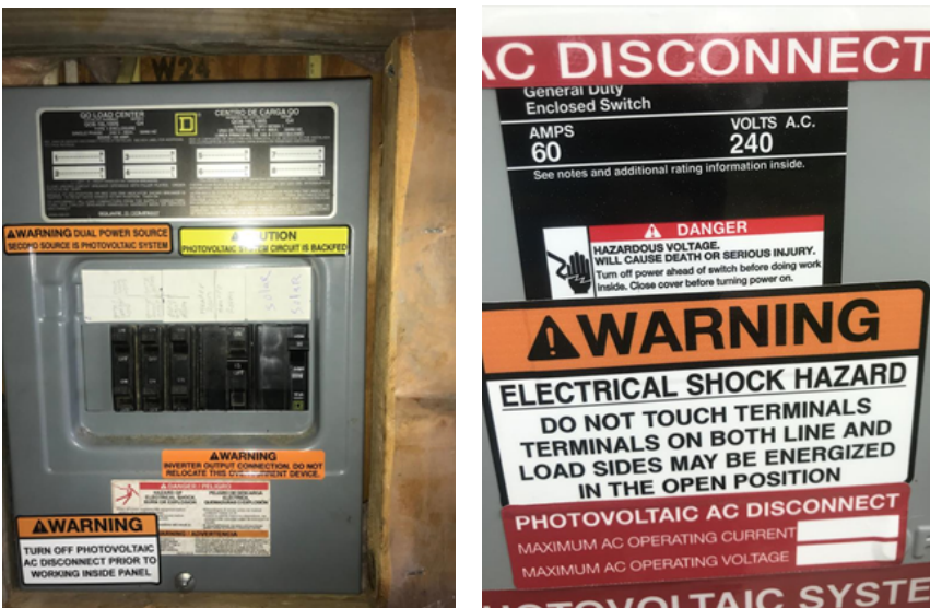
Photo 11: AC disconnect/load center manufacturer's label obscured: NEC 110.21
